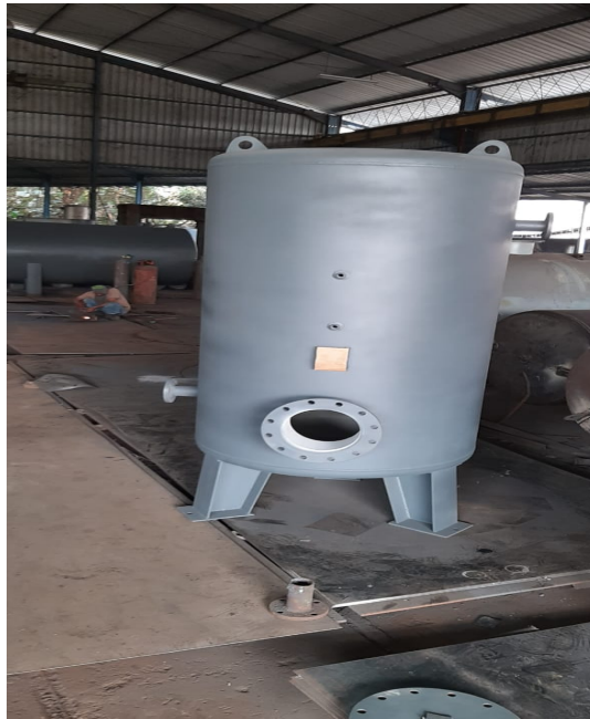
Gambar 1. Water Pressure Tank
